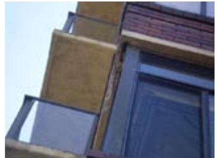
Corrosion of posts, spalling slab
