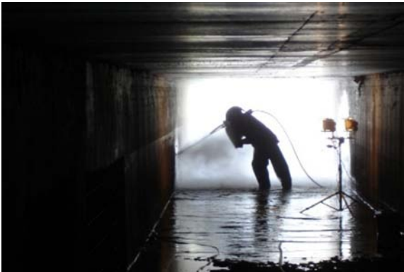
The Preservation Technologies team used hydrodemolition to expose and clean the steel
