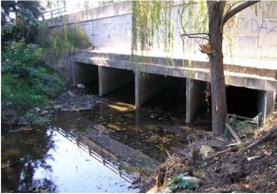
Carbonation had combined with low concrete cover to cause severe concrete deterioration
