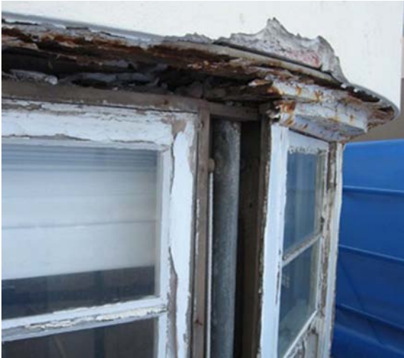
The curved lintel area had badly deteriorated
