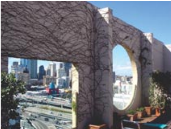
3m high parapets required structural strengthening
