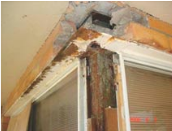
The remedial team exposed the structural steel to inspect the corrosion before repairs
