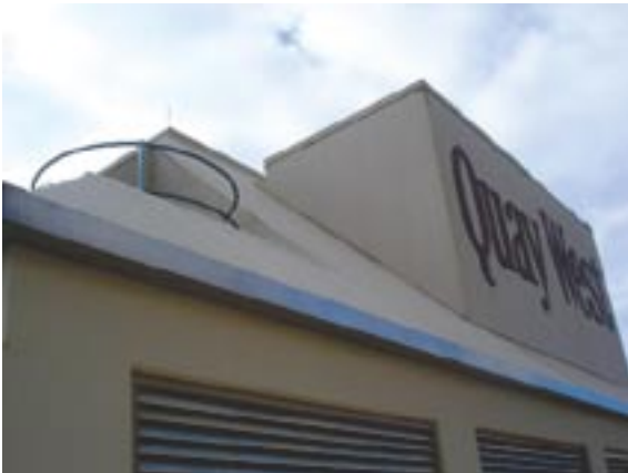
All roof areas had to be accessed for coating and waterproofing works as well as metalwork replacement
