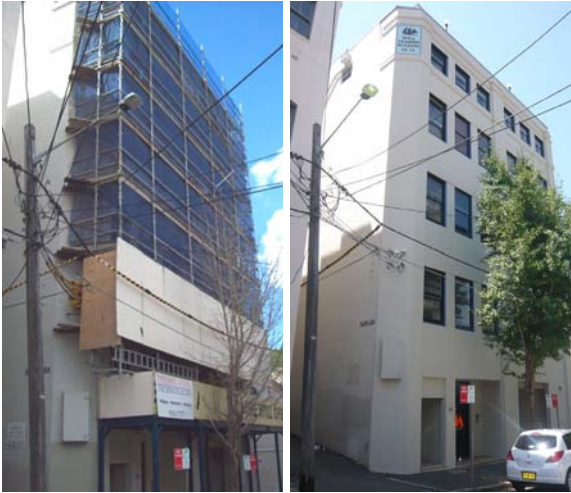
Left: Access to the southern elevation, and Right: The southern elevation repaired and coated
