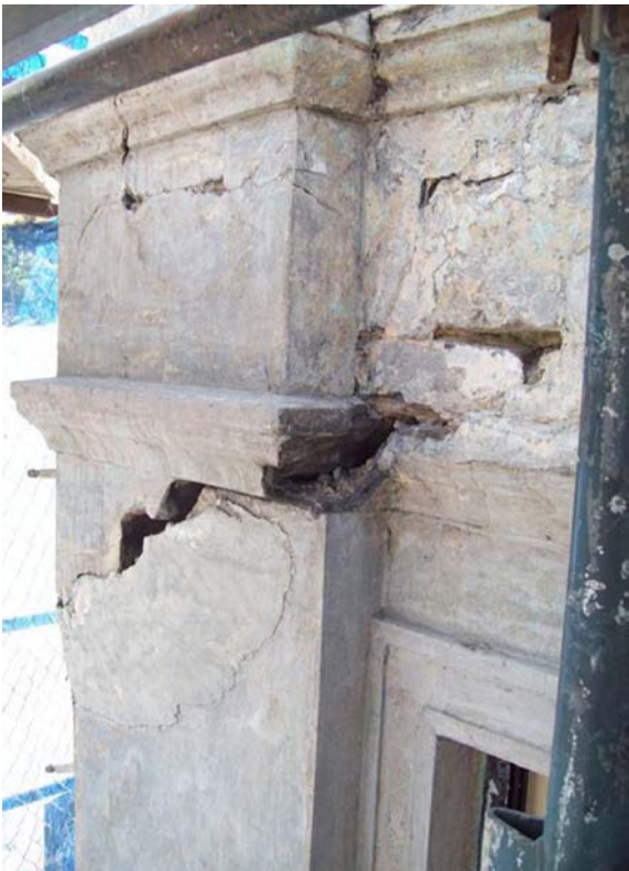
After major preparation work internally, the lintel had to be completely rebuilt
