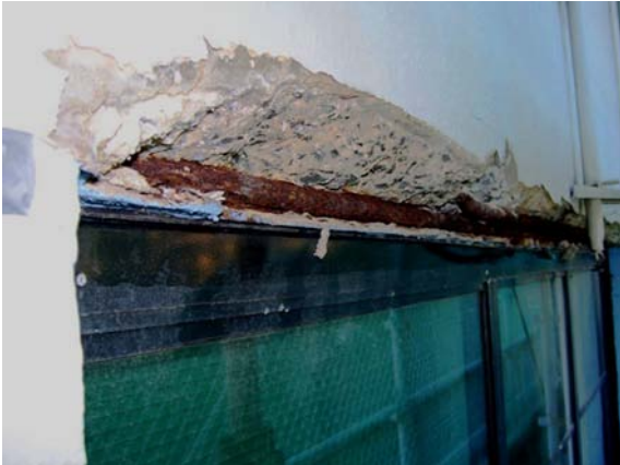
This was typical of the deterioration of the lintels
