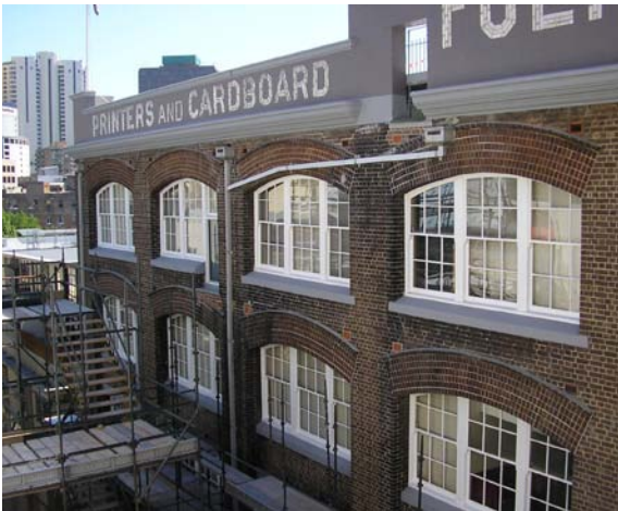
The team refurbished the parapet including glazed tiles, restored the windows and repaired and protected the lintels and sills
