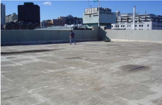
The existing PVC membrane needed replacing
