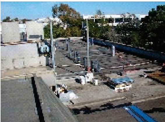
The old membrane had to be stripped and the new system applied in sectional areas
