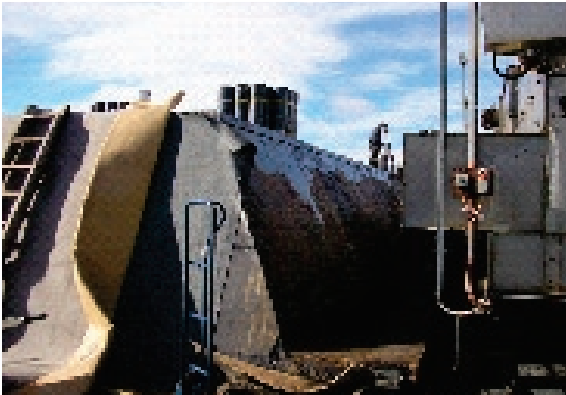
The membrane had to be applied to sloping roof areas and under low level plant installations
