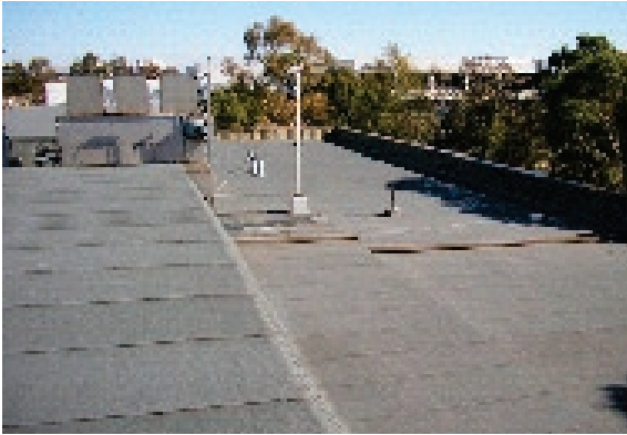
Project completed, with the torch-on membrane applied to all elements of the roof
