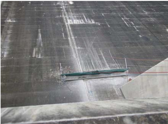
The work platform hangs down the dam face with a net underneath to catch dangerous "fall-out"
