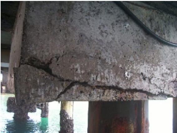
Reinforced concrete pile caps had deteriorated badly at tidal level
